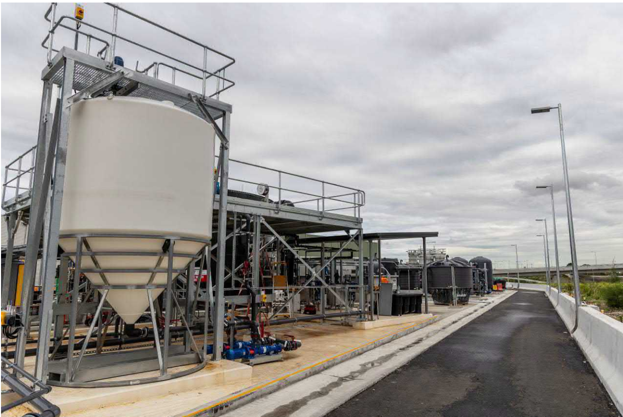
Figure 2-1 Operational Water Treatment Plant, St Peters April 2022
