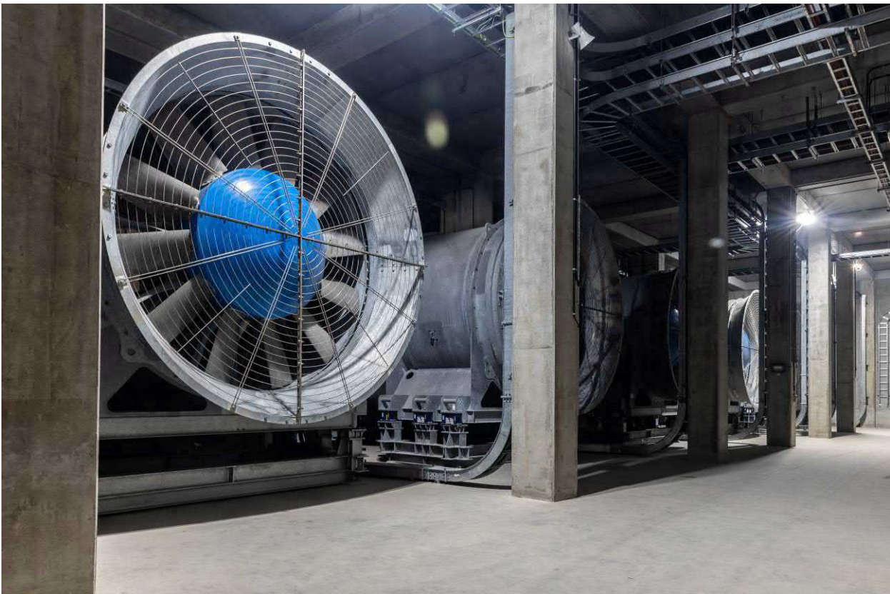
Figure 2-5 Ventilation building axial fans, St Peters April 2022
