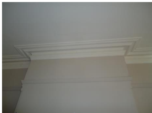
Plate 67 Interior of 44 Campbell Street indicating the preservation of the cornice and picture rails.
