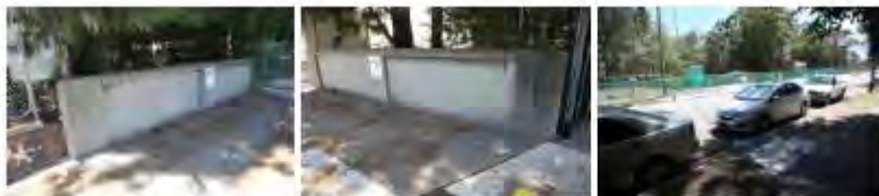
025_MACDONALDTOWN_STORM WATER_CHANNEL_2017 1/8 ISO 640 2017/02/09 12:10:48 026_MACDONALDTOWN_STORM WATER_CHANNEL_2017 1/8 ISO 640 2017/02/09 12:11:07 027_MACDONALDTOWN_STORM WATER_CHANNEL_2017 1/8 ISO 640 2017/02/09 12:11:18
